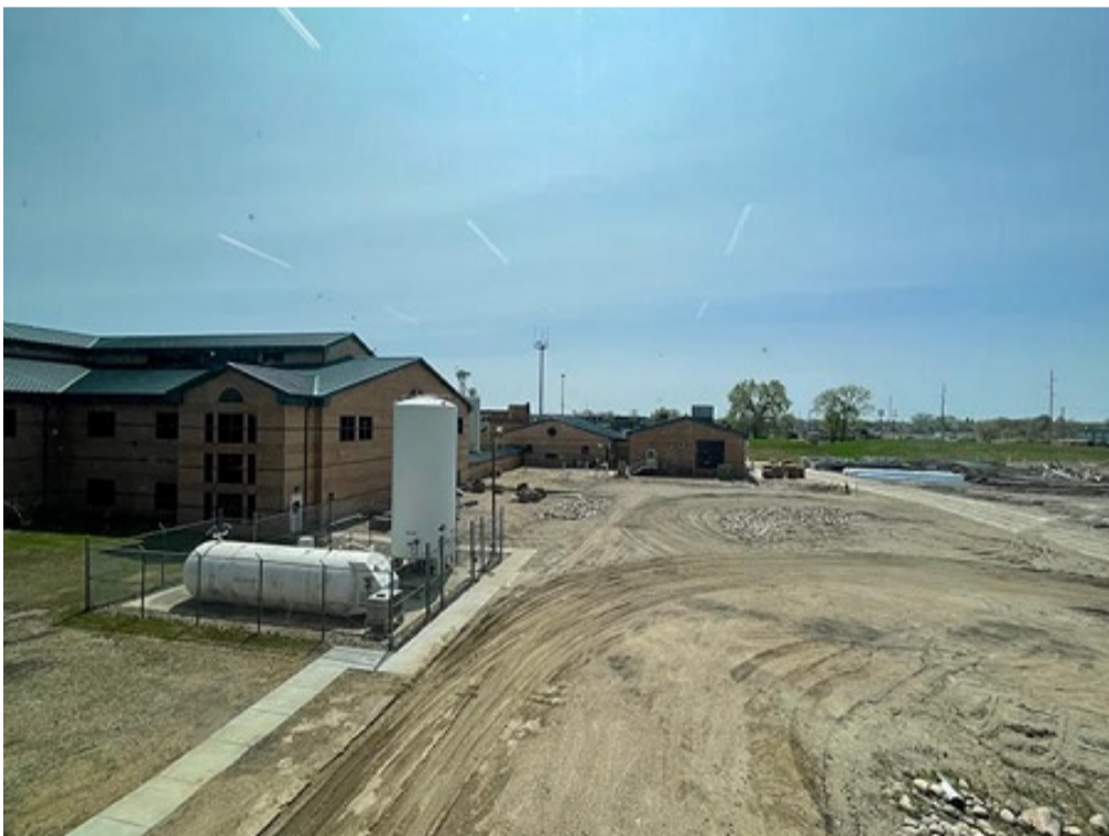
The existing plant is to the south of the new dewatering building.
